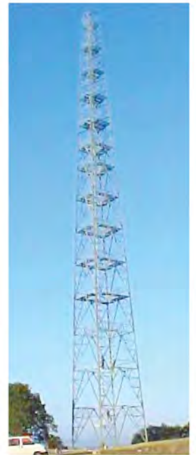
Lattice type transmission towers of various heights from 30 m to 70 m.
